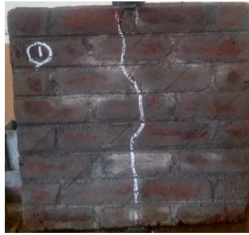
Figure 8: Failure of Specimen with Horizontal Joints
